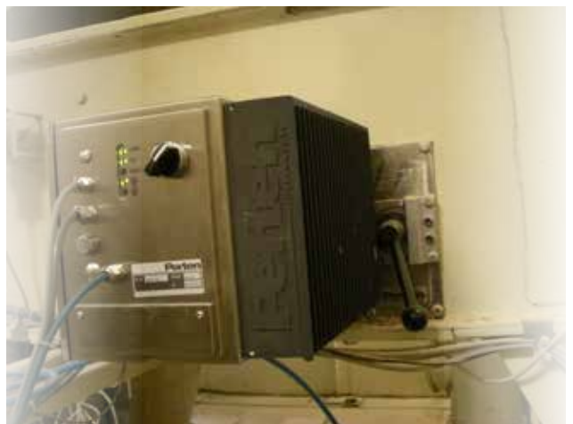
Feed Measurement of feed pellets in a chain conveyor, for control of fat spraying.
