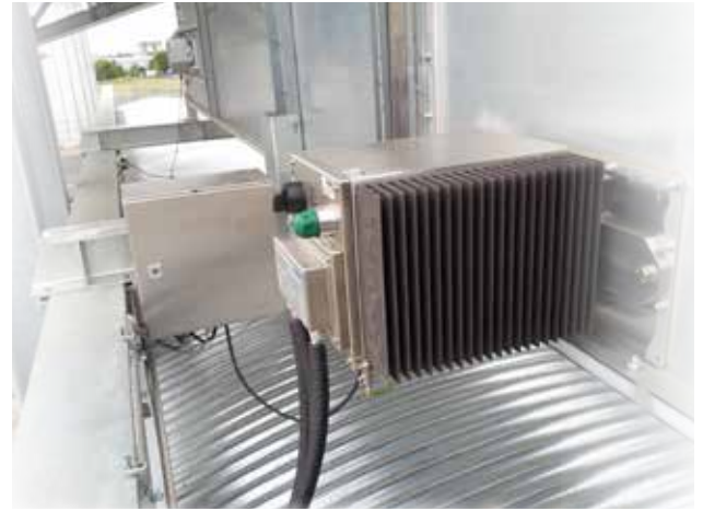
Grain Installation at a ship loading facility for continuous measurement of grain.
